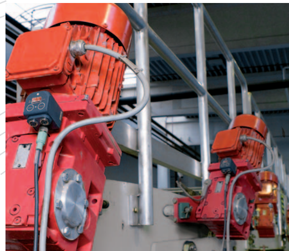
Machinery monitoring by means of FAG SmartCheck
